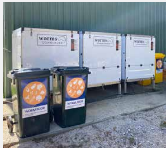
The units are installed at the Whitemark Waste Facility. Photo: Sabrina Carter, Flinders Council.
