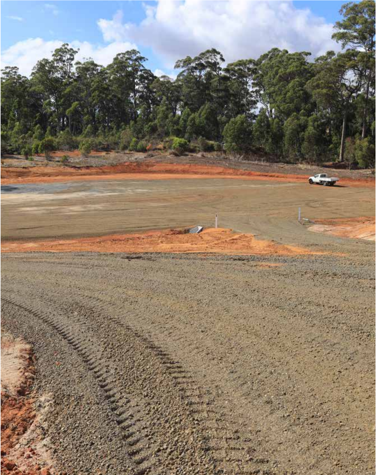
Scottsdale Waste Transfer Station's new green waste pad. Photo credit: Dorset Council
